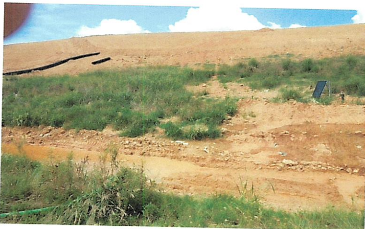
Photo shows area G toe is wet and pumps are pushing liquids to the other side currently to inside ~B pumping which runs to frac tanks. The culvert is blocked and this area is planned for closure top liner system. Run off is not possible today to the pond and confinement & management required and considered mitigation until pending closure work for this section.
