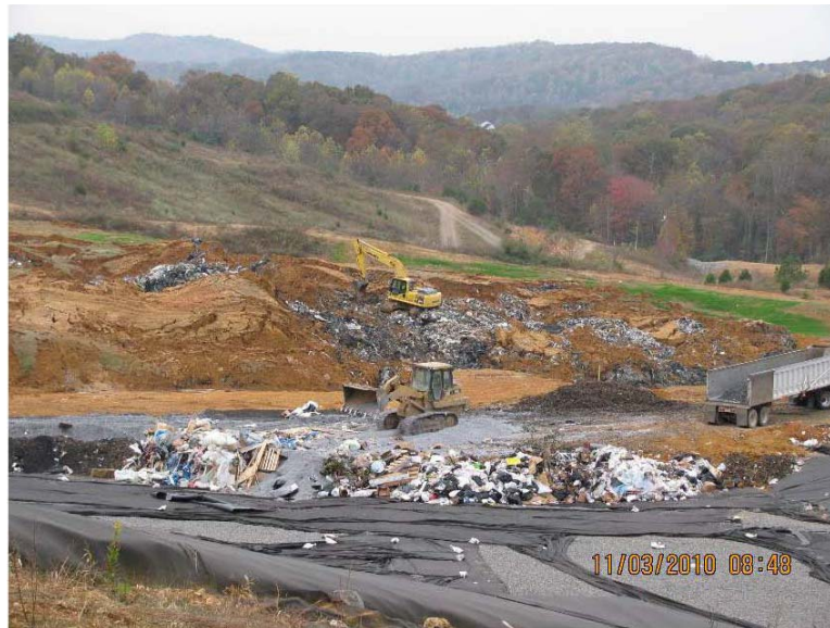
Figure 3. View of the Failed Material at the Toe on 3 November 2010
