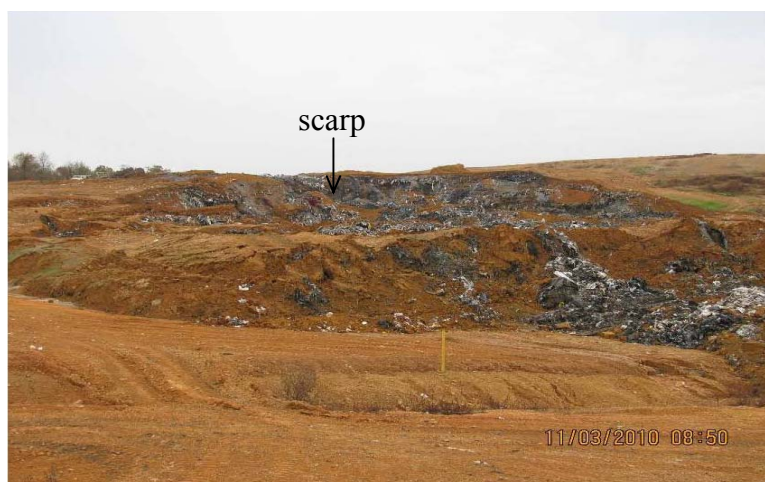
Figure 2. View of the Failure Area from the Toe on 3 November 2010
