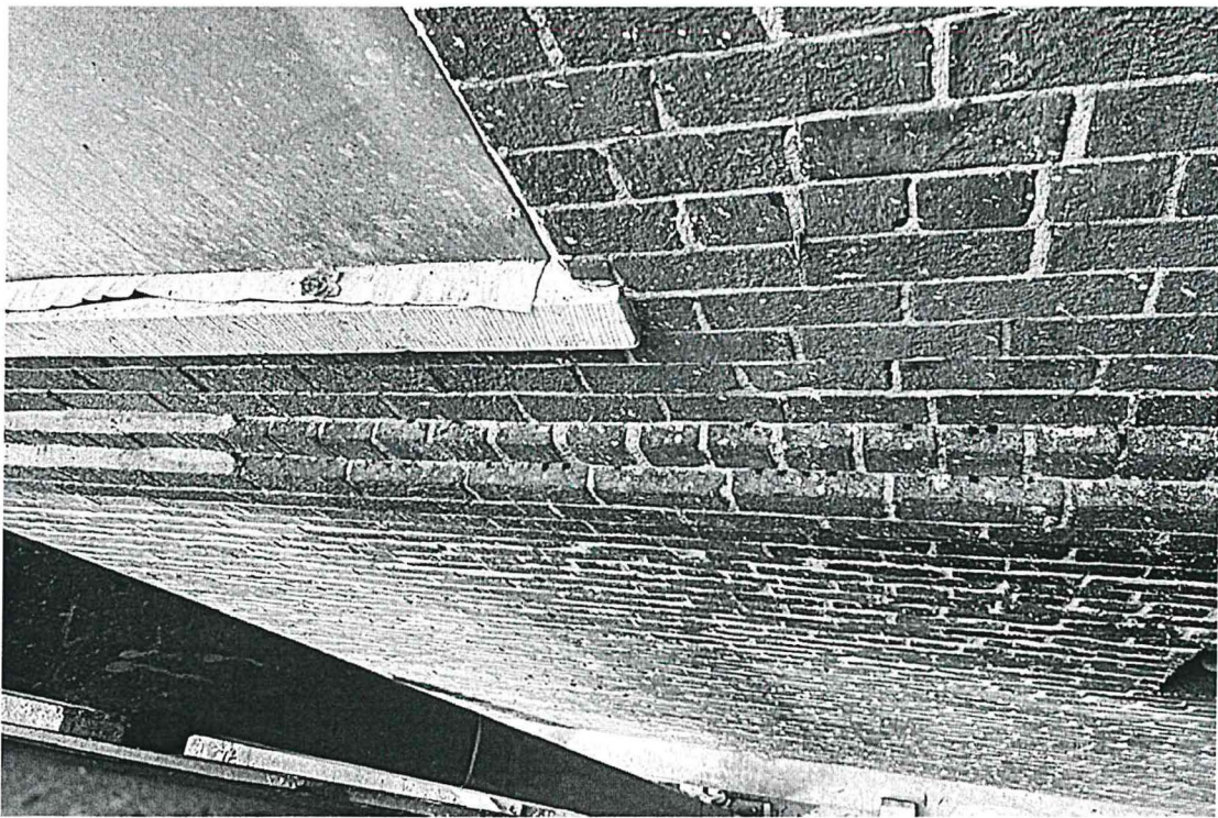
Loudon County Courthouse, Change Order No. 6, $3,717 Cost Item Examples of brick ledge areas with exposed corings due to loss of mortar wash.
