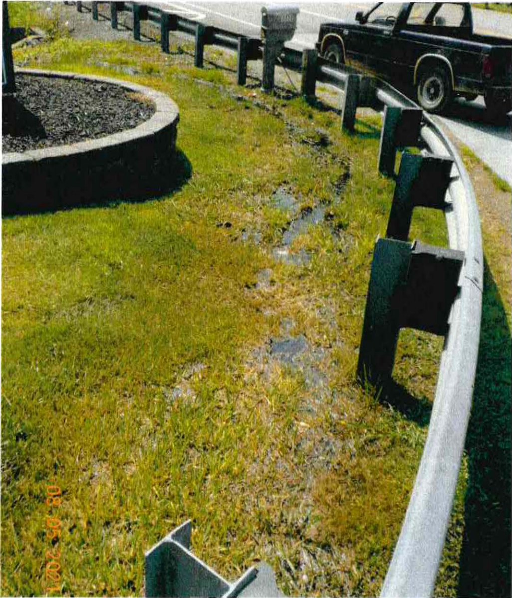
Spring flow is directed to follow the curve of the road/driveway into the ditch (upper left).
