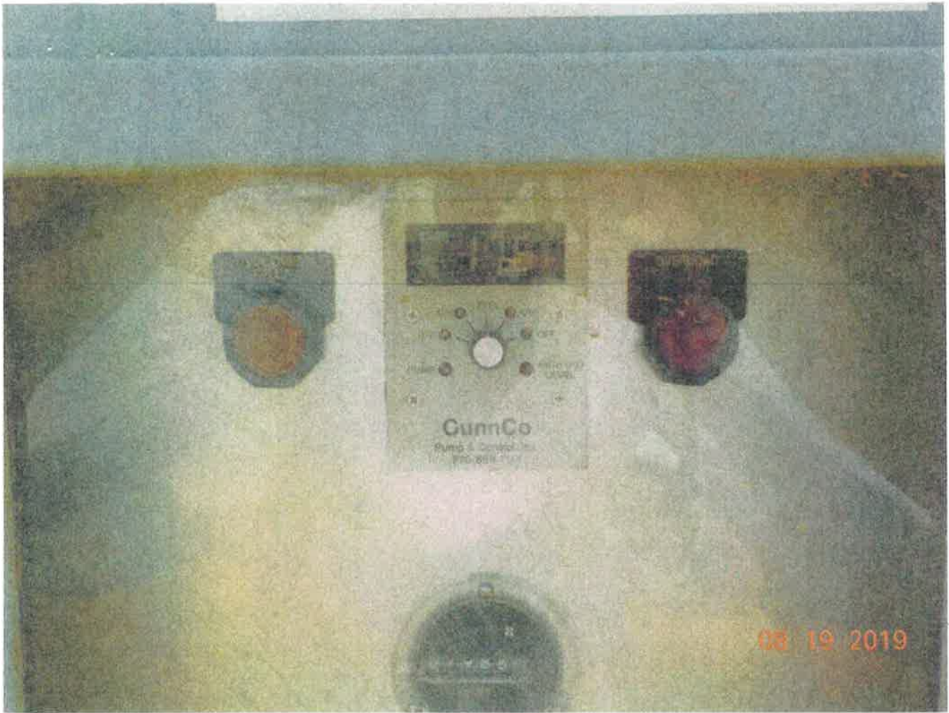
Leachate level at sump = 11.6". Compliance level = 12".
