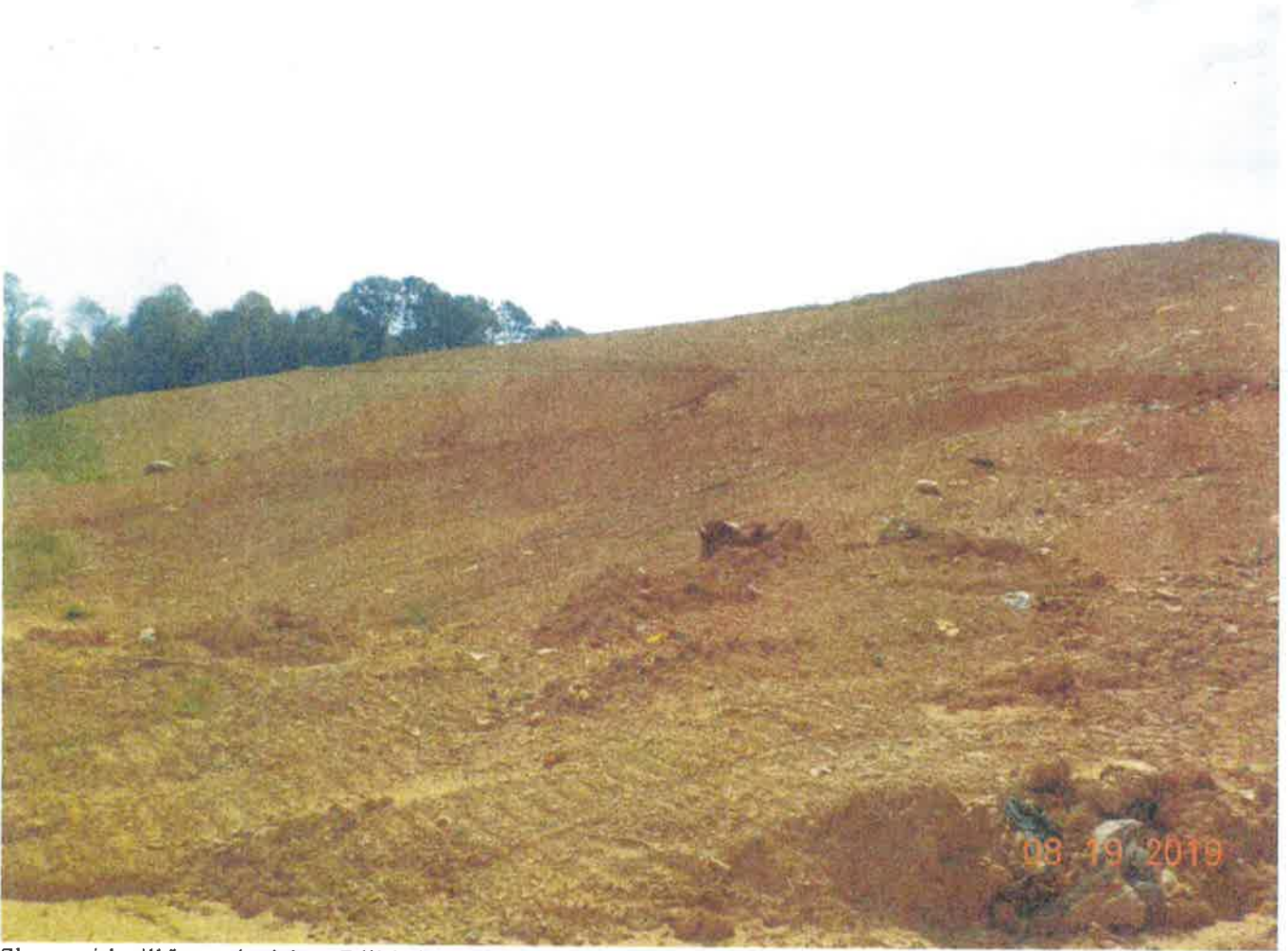
Slope with rill/berm incision. Rill is in center of frame.
